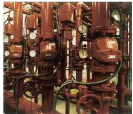
Multiple Wet Pipe Risers, MTS, Bangkok
