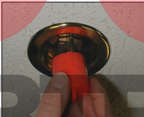
Figure 2: Sprinkler cap being removed from a pendent sprinkler.
