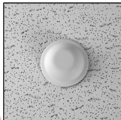
Concealed Sprinkler and Adapter Assembly (Protective Cap Removed)
